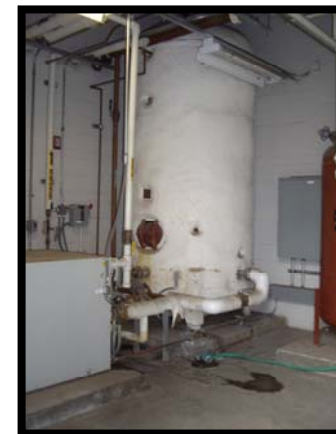
(OLD) heating boilers
